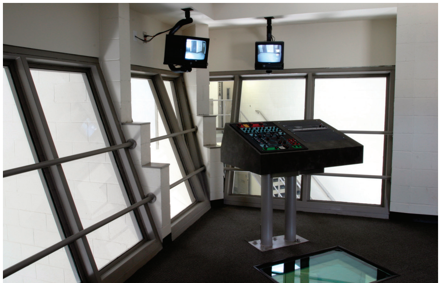
The elevated control tower provides sightlines to all the jail's housing units. The control panel is mounted on a pedestal to make room for the view window in the floor, allowing an officer to view the sallyport below.
