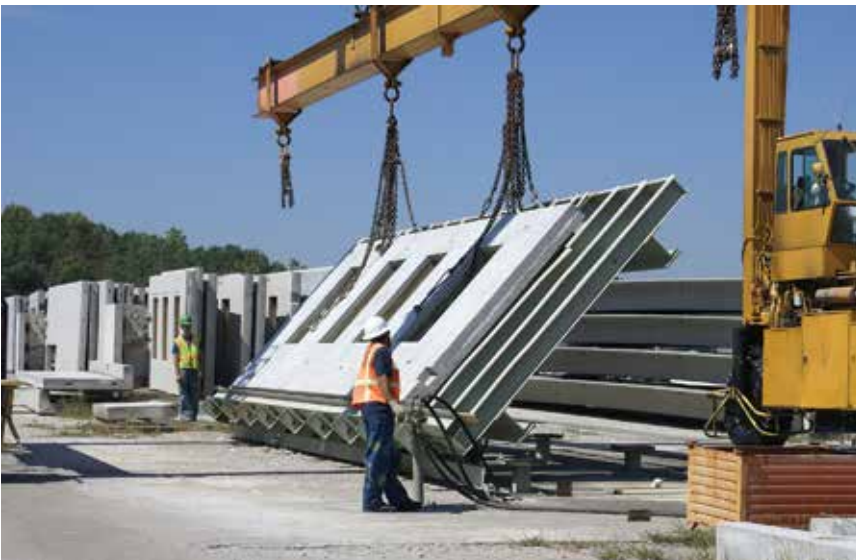
First-floor panels features a variety of windows cast into the panels, with interior insulation running up against the penetrations. Photo: Metromont Corp.
